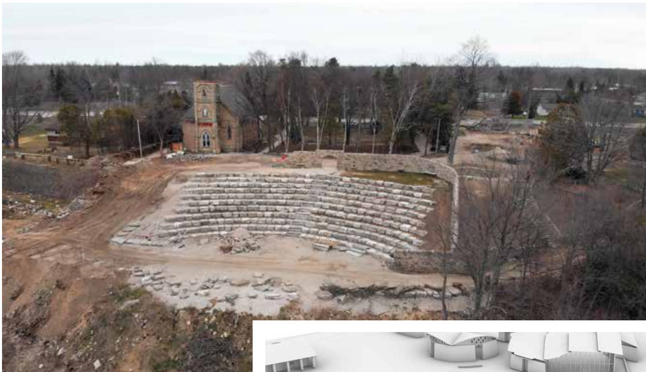
LEFT AND BELOW Work to complete the amphitheater and surrounding drystone walls is under way.
